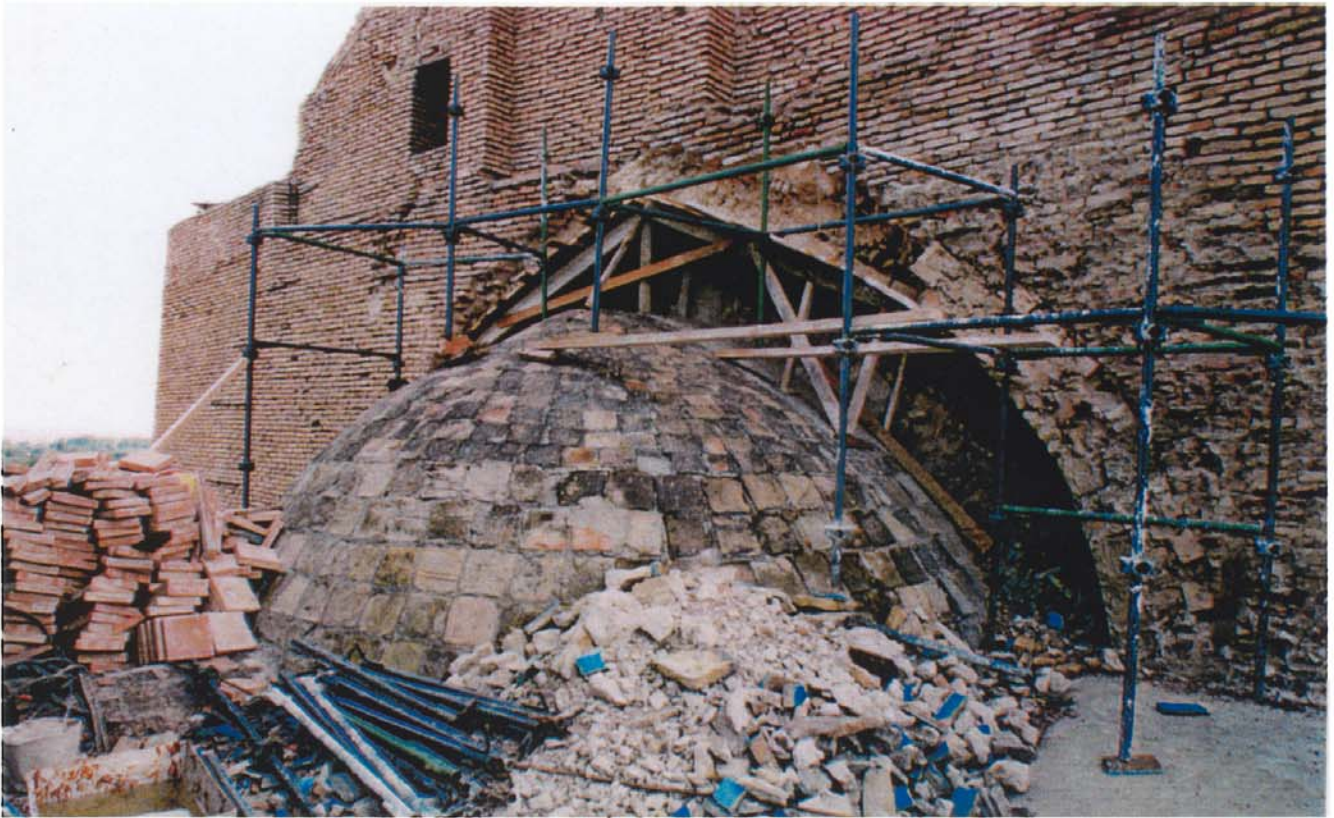
Above: Before restoration of a secondary dome.
